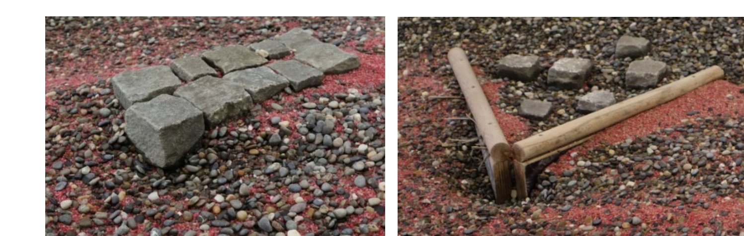
Figure 5: Examples of local scour after HQ100
